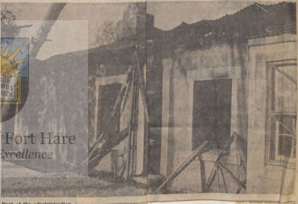
Part of the administration building of Lovedale Teachers' Training College, formerly the principal's house, which was destroyed in a fire early on Monday morning. The building and contents were valued at about R80 000.
