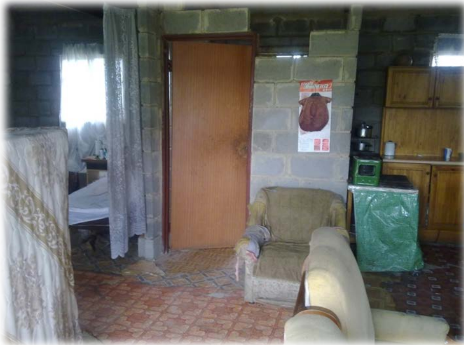
Picture 8. (The house is not properly built that the bricks in the toilet easily collapse)
