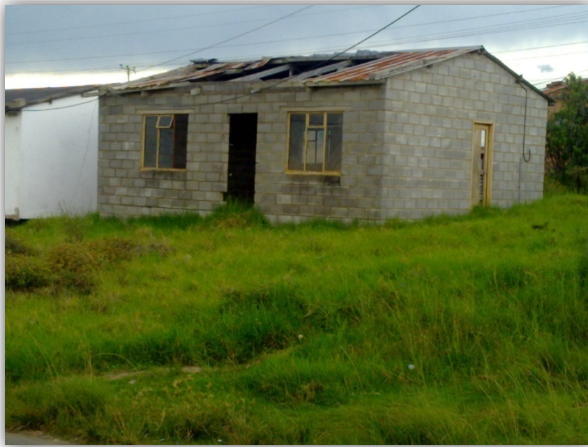
Picture 5. (The RDP house with a roof that is blown away by wind)
