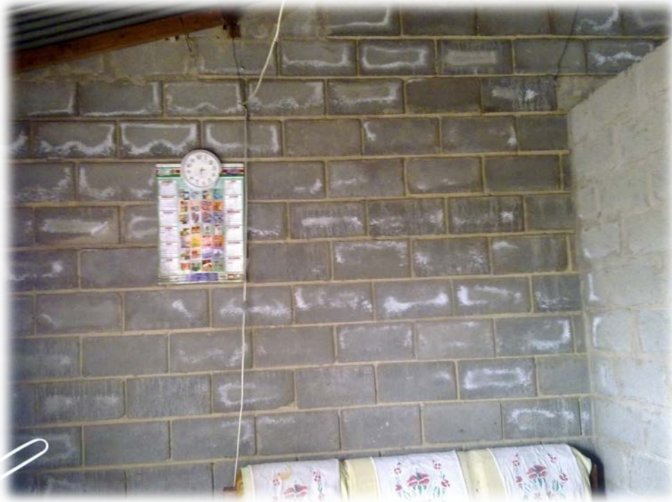
Picture 7. (The wall is easily penetrated by water)
