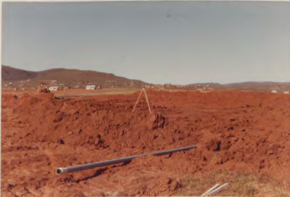
Drainage pipe laid and first layer of dam wall ready for compaction
