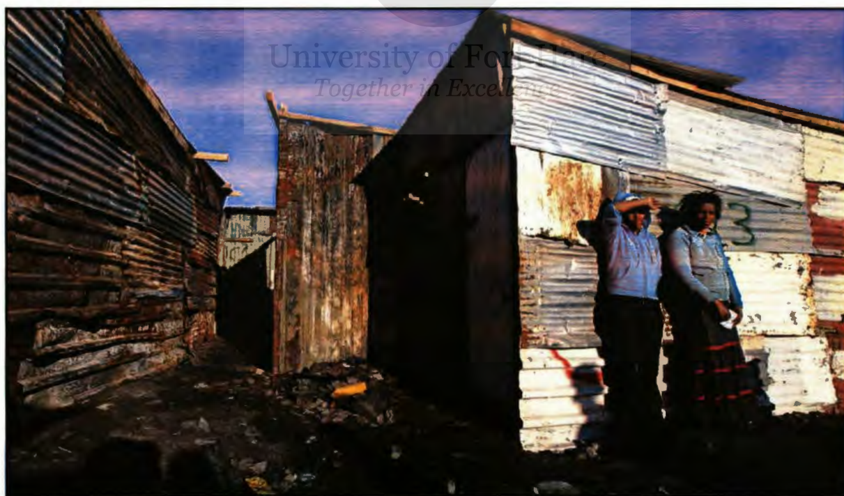
Figure 19: Image 16- Poor South African housing facilities
