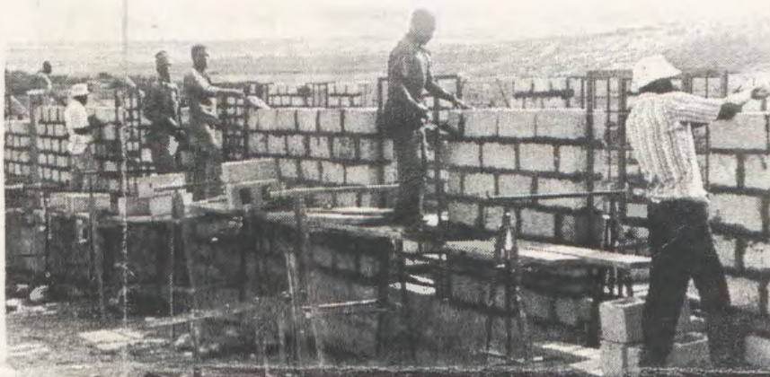
Renovations, alterations and extensions were the mainstay of the small building contractors after the coup.
