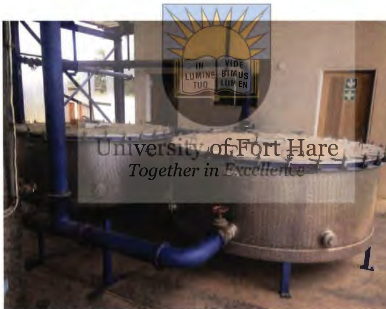
Figure 3.7: Picture of the sawdust filters
