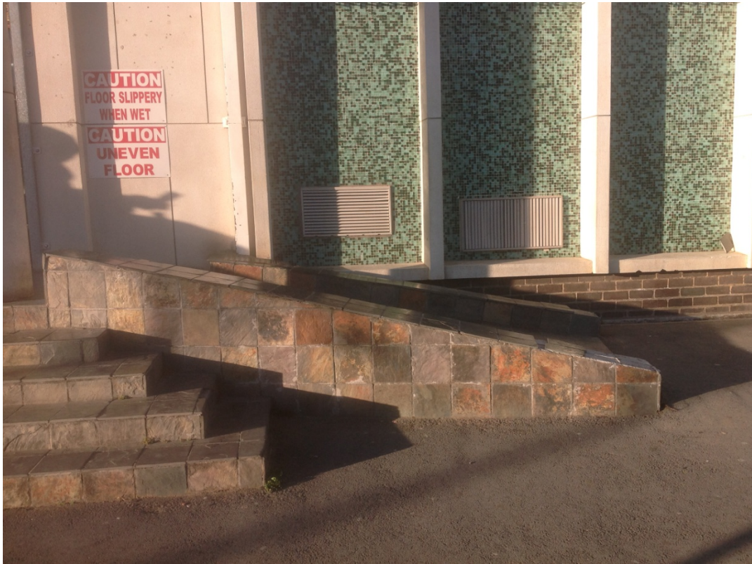
PLATE NO. 14: Ramp (King Williams Town Library)
