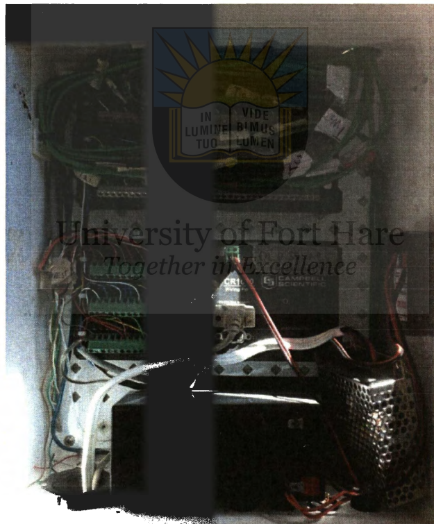
Plate 3.3: Data acquisition system (A): the passive solar house sensors
