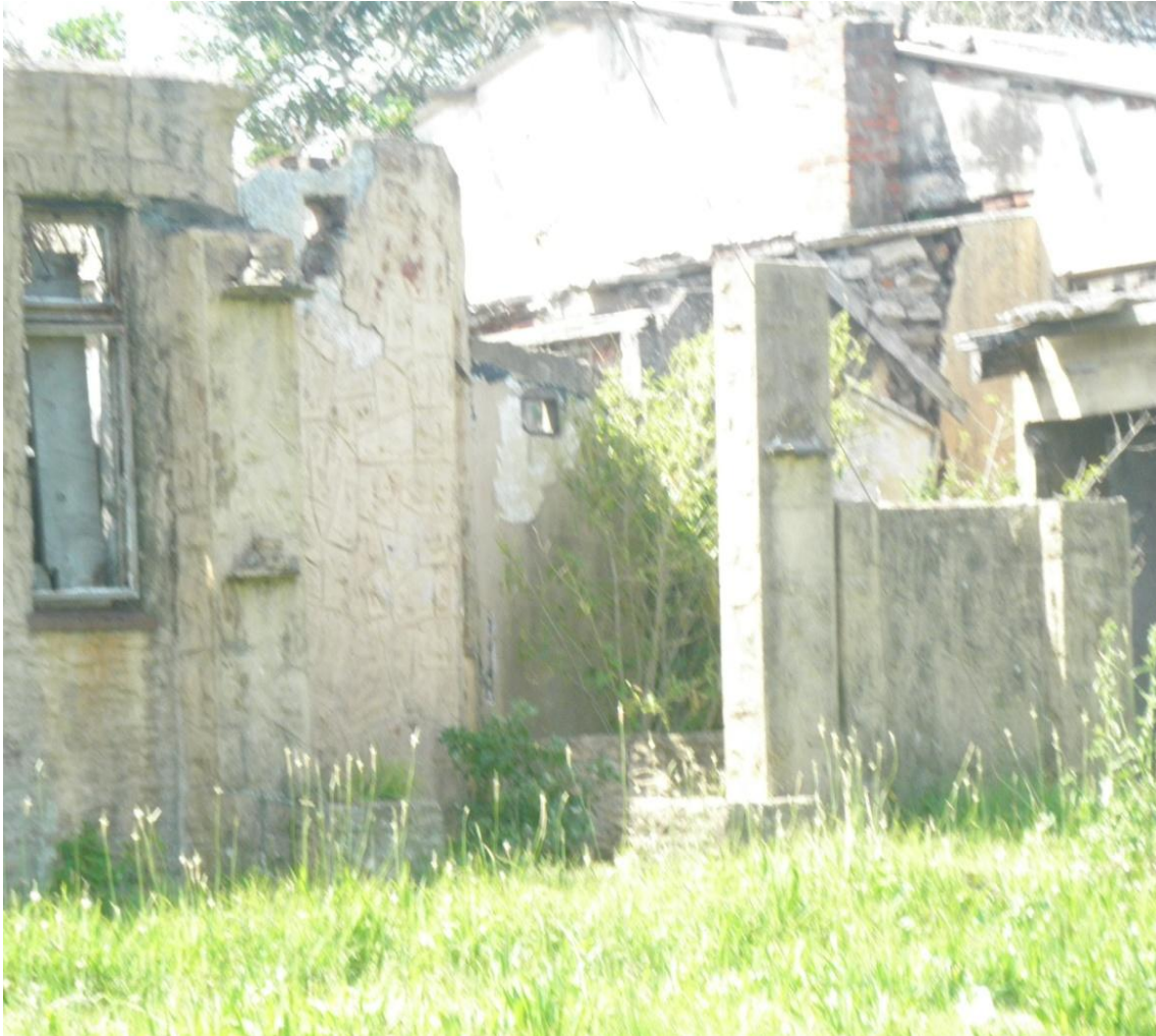
Picture 3: A dilapidated house in Cocobana
